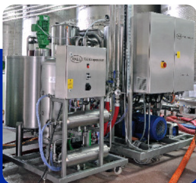
Figure 1: Oenofine XL Dosing Skid
